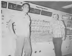
H3AR Panel Operators in the Refining Operations Center (l to r): E. Boekhoud and A. Croes. Not in picture E. Croes.
